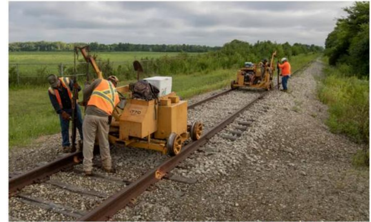
A crew for Utah's A & K Railroad Materials removes railroad spikes Wednesday on the Nickel Plate Line. RobertScheer
